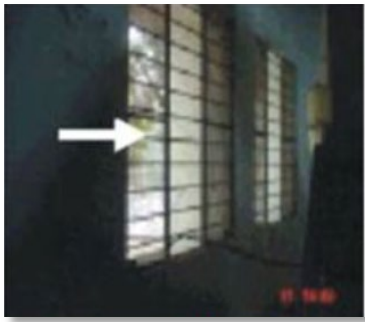
Broken glass at the window
