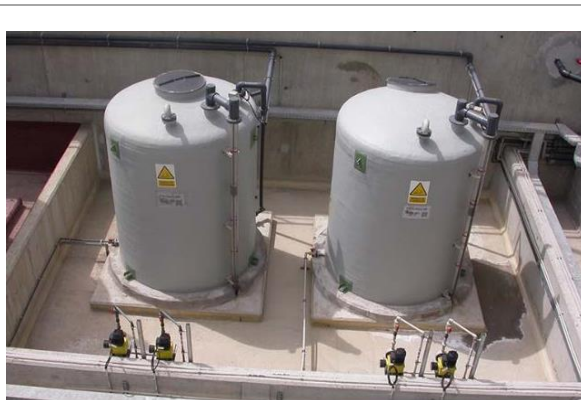
Fig. 4.3.3. Chemical treatment tanks/cooling tanks
