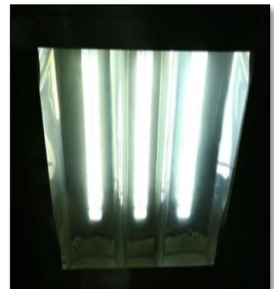
Fig.6.3.26.Covered lights in the production area
