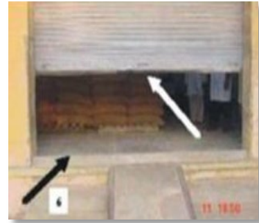
Gap in between shutter and floor
