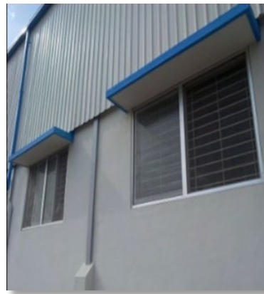
Fig.5.3.25. Nets and mesh on windows to avoid pest entry
