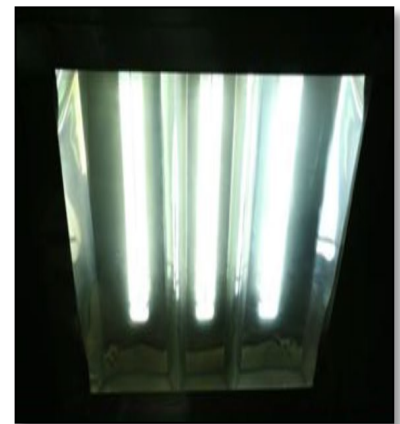
Fig.5.3.26. Covered lights in the production area
