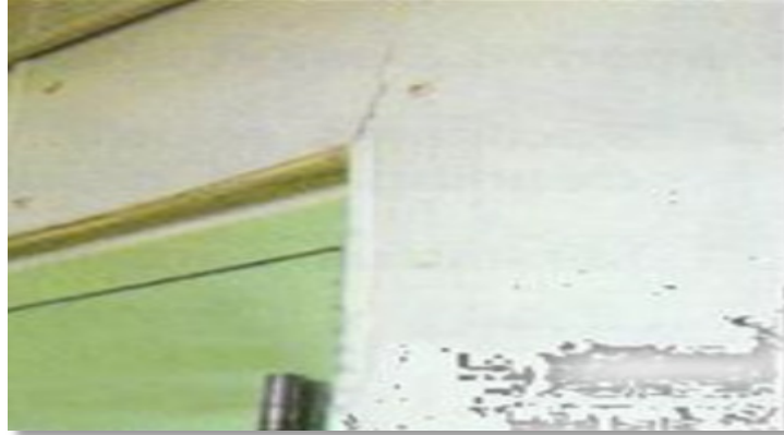
Fig.5.3.17. Avoid Cracks on walls as it allow bacteria and moulds to accumulate
