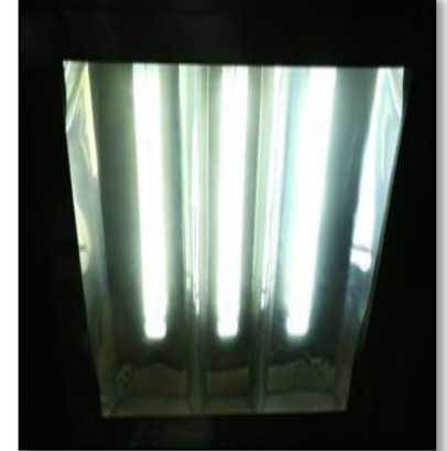
Fig.6.3.26. Covered lights in the production area
