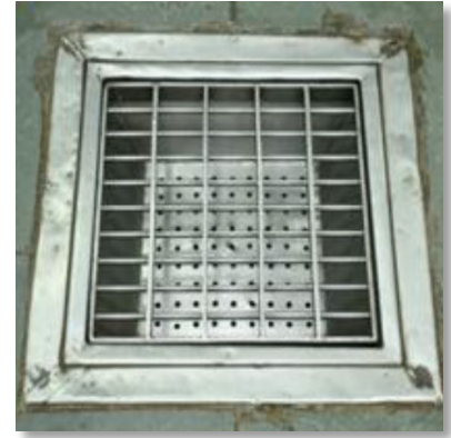
Fig.6.3.23. Covered drains to prevent insects and rodents
