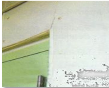
Fig.6.3.17. Avoid Cracks on walls as it allow bacteria and moulds to accumulate
