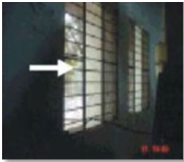
Broken glass at the window
