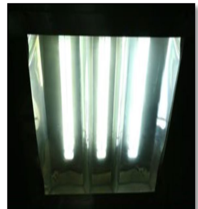
Fig.6.3.26.Covered lights in the production area
