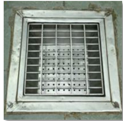
Fig.6.3.23.Covered drains to prevent insects and rodents
