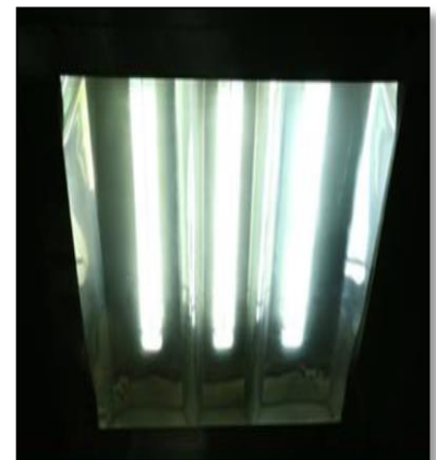
Fig.6.3.26.Covered lights in the production area
