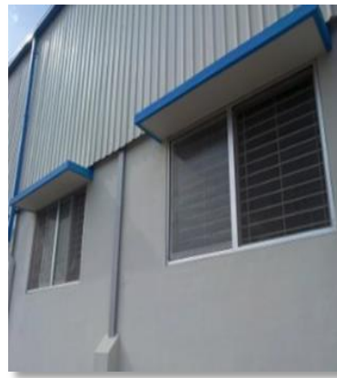
Fig.6.3.25.Nets and mesh on windows to avoid pest entry
