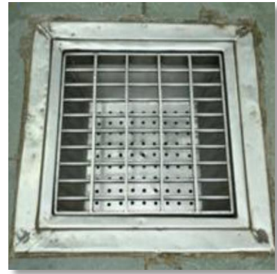
Fig.6.3.23.Covered drains to prevent insects and rodents
