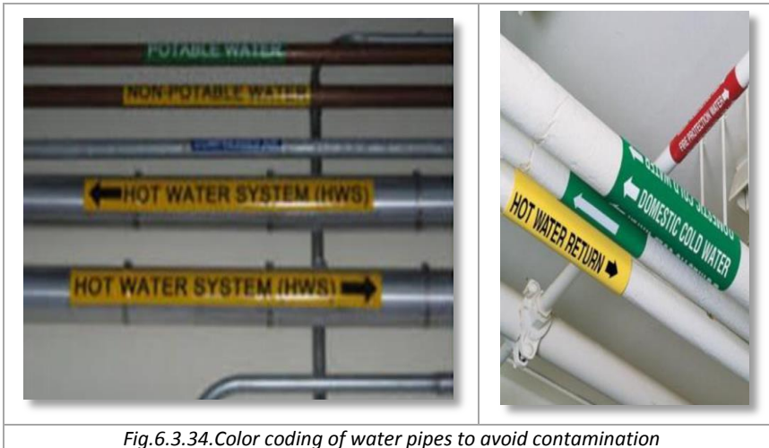
Fig.6.3.34. Color coding of water pipes to avoid contamination
